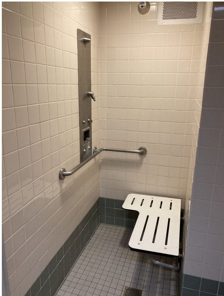
Image 25: ADA solitary confinement shower at Washington Corrections Center for Women (WCCW).
